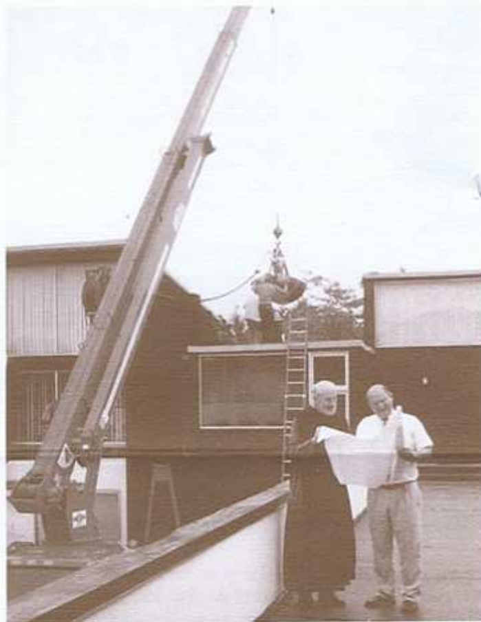
Fr. Martin and Bob Gill look to future repairs of the link between the chapel and the monastery buildings while work continues on the roof and sides of the East Building.
