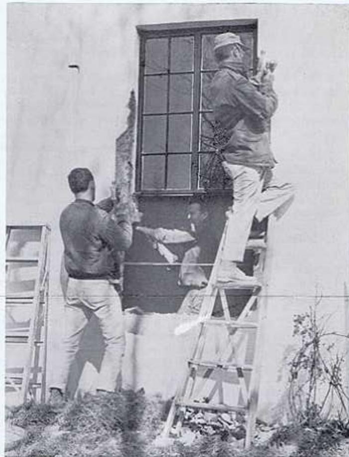
REMODELING at St. Joseph's guesthouse — enlarging a window in the new living room area. Rocco Picarazzi, who appears inside the window has been building and rebuilding at Mount Saviour since the earliest days.
